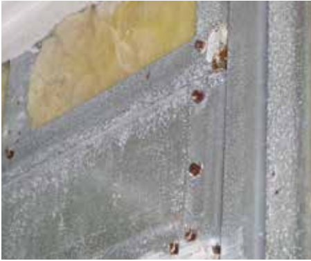
Image 1: Corrosion of the studs and fasteners on a 7-story concrete and metal framed building in a hot-humid climate, 7 years after the building was completed. The exterior water and air control layer of this building was a mechanically-fastened building wrap that was not detailed to be sufficiently airtight, nor was it sufficiently water-vapor impermeable to counteract high moisture drive from the exterior to the interior.
